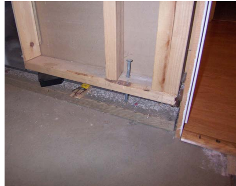
Hanging wall on concrete slab floor.
